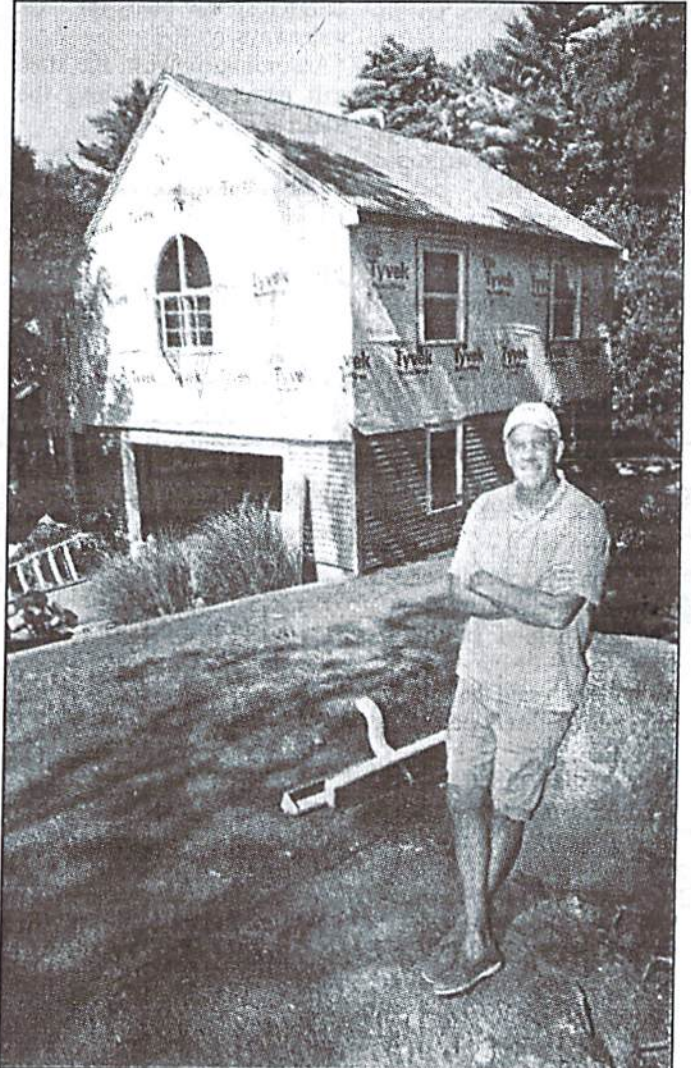
STAFF PHOTO/CHRIS BERNSTEIN Builder Tim McCluskey with a recent addition and remodeling job.
